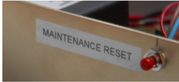
Figure 12 – MAINTENANCE RESET button
